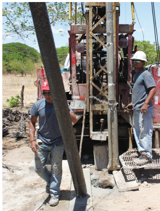
A well-drilling rig such as this one will be used to tap into a water source 420 feet below ground.
